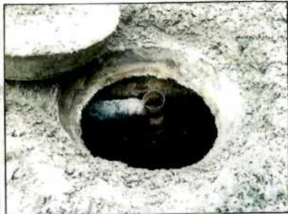
12.1 Item 2(Picture) Tank level low, outlet baffle OK
