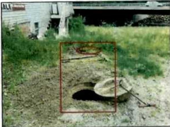
12.1 Item 1(Picture) Septic tank location
