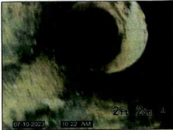
12.1 Item 5(Picture) Line from home to tank
