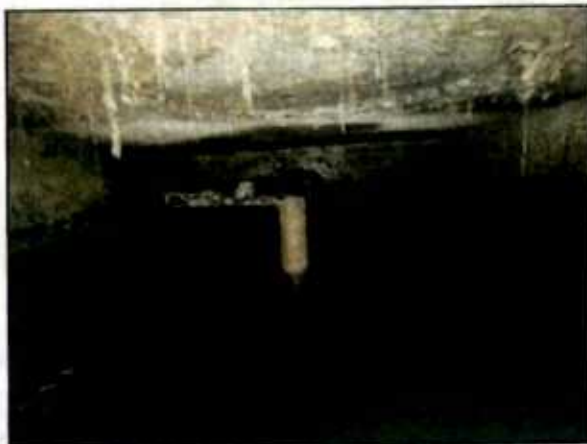
12.1 Item 3(Picture) View of Inlet baffle
