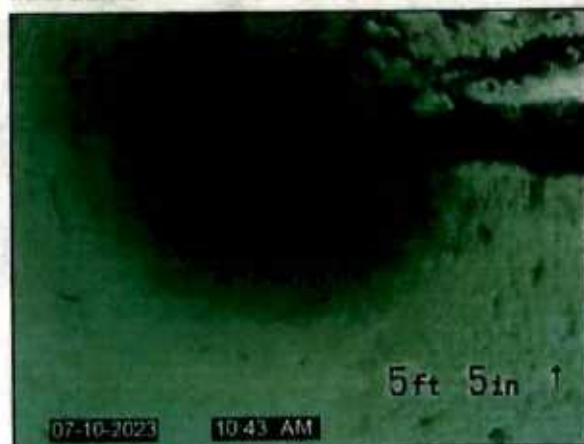
12.1 Item 9(Picture) Line scoped from tank to leachfield
